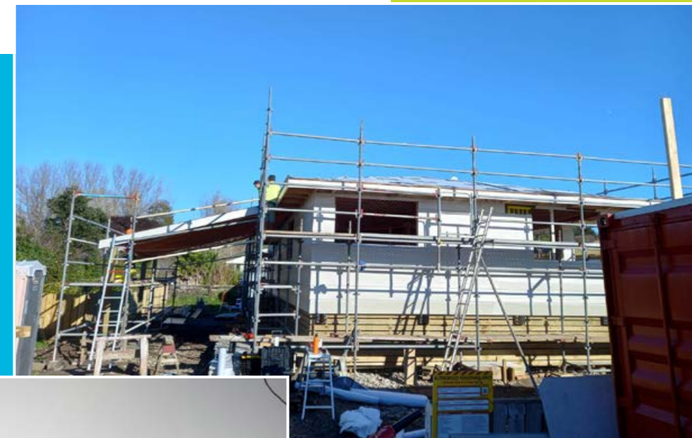
Construction of a new home for a Habitat for Humanity Taranaki Progressive Home Ownership partner family. A housing dedication was held for the whānau this October (right)
