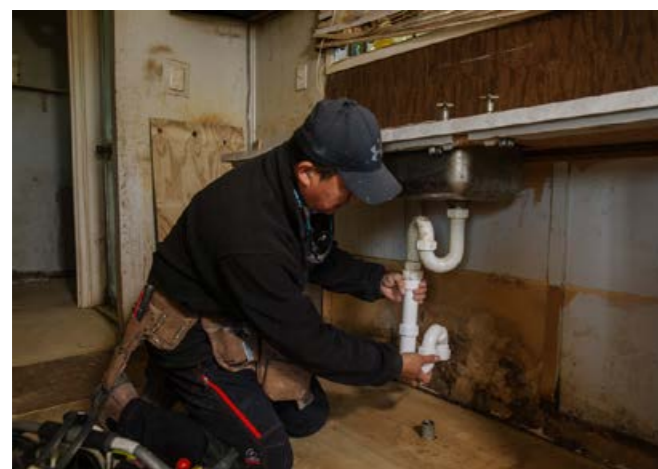
Habitat Build Team member Hoon Jee carrying out essential repairs to the kitchen.
