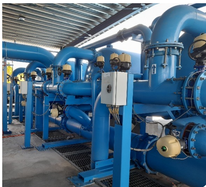
Figure 5 - Waiwai water treatment plant, Ba province
