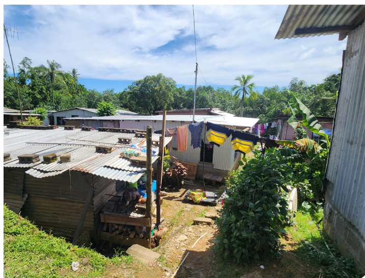
Figure 15- Cement blocks placed to hold down the roof instead of proper nailing and strapping.
