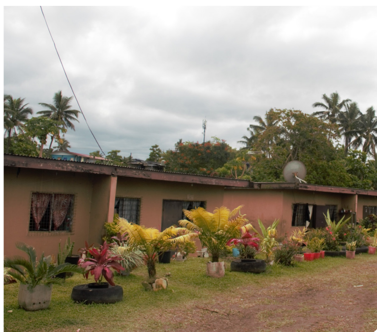
Figure 7 - PRB Estate located in the Nasinu area. Rotting fascia board and missing louvre blades visible in the PRB Flat on the left of this photo
